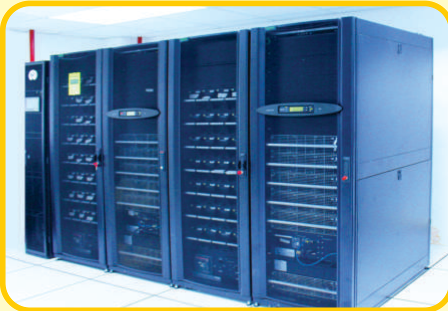
Data Center at the National Statistics Office
